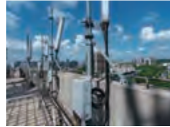
(5G Mobile Base Station)
