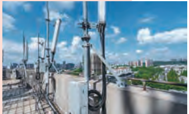
5G mobile base station
